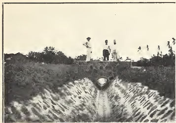
Fig. 2. A culvert over a large drainage channel at La Chorrera, Republic of Panama. This ditch was paved with inverts and the sides faced with stones set in cement.
